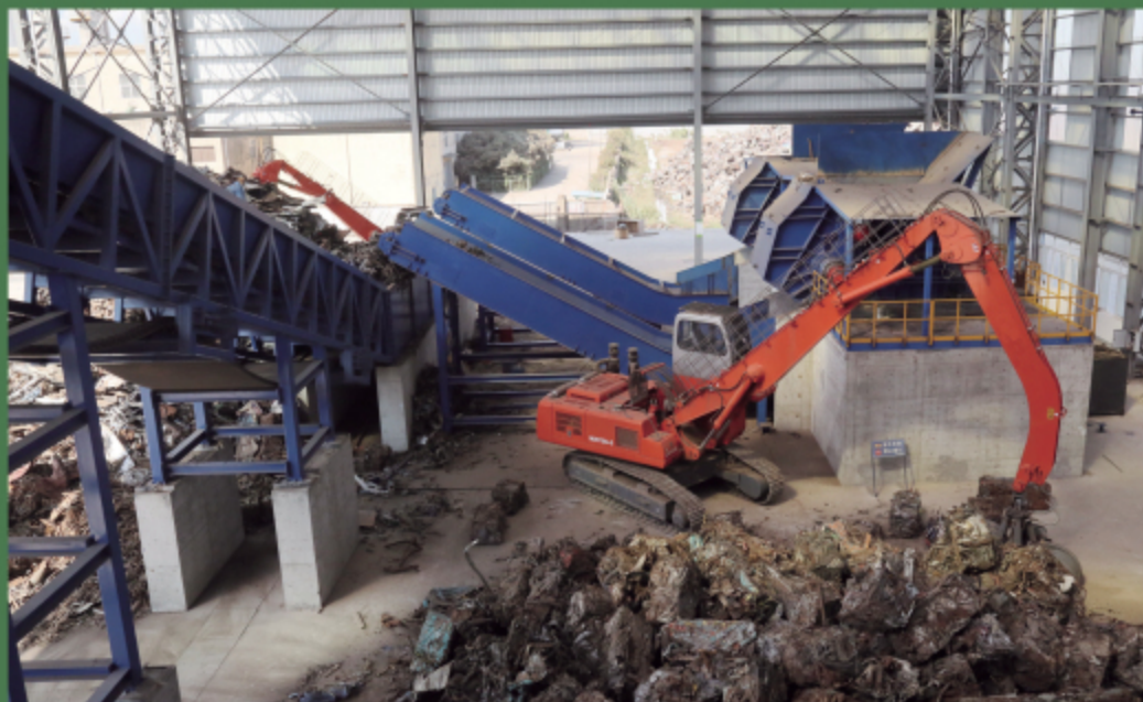
中再生纽维尔向沙钢提供的两台废钢预破碎机正在处理废钢压块，该生产线为国内首条进口预破碎机生产线。 The two sets of pre-shredders provided by China Recycling Newell to Sha-steel Group are dealing with the scrap steel bales. It is the first imported pre-shredder production line in China.
