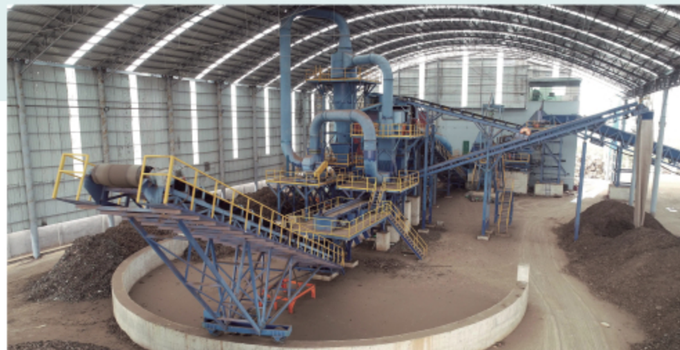
84 SXS型 4000匹马力废钢破碎生产线实景 Reality images of 84 SXS scrap shredding production line with 4000HP
