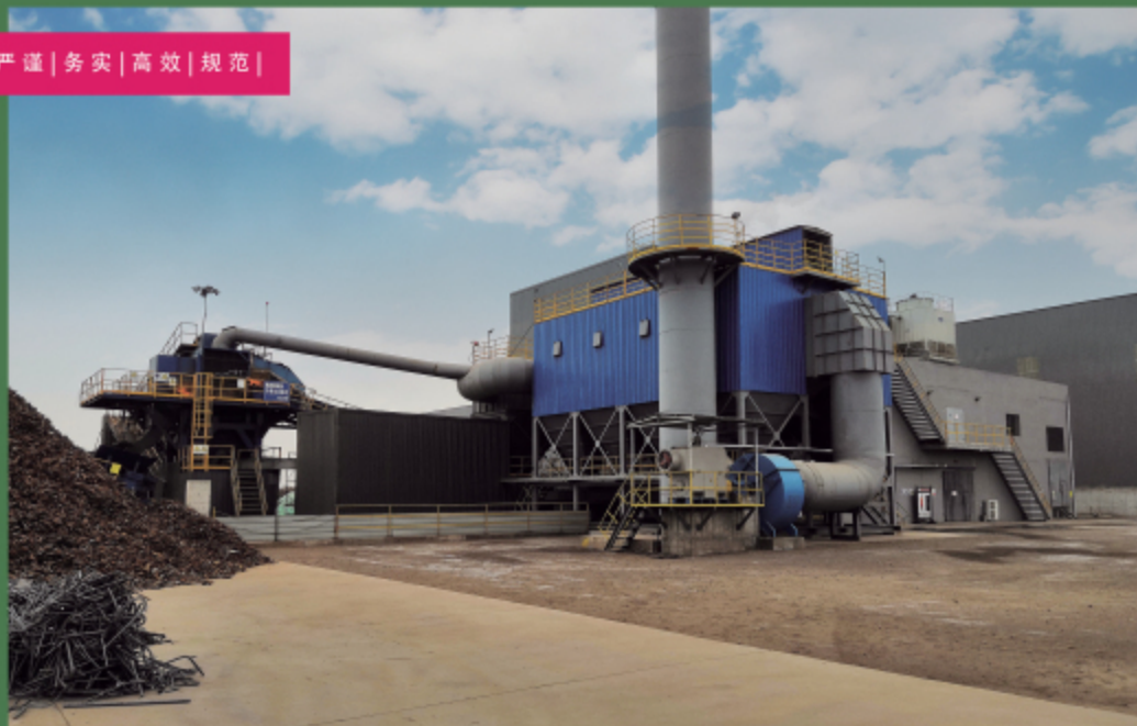
宁夏4000匹马力破碎线，设备运行稳定可靠，防噪音及除尘效果理想，得到客户和环保部门高度认可。 The shredder production line with 4000HP of Ningxia Project, runs stably and reliably with significant effect of sound proof and dust removal, which are highly recognized by customers and environmental protection department.
